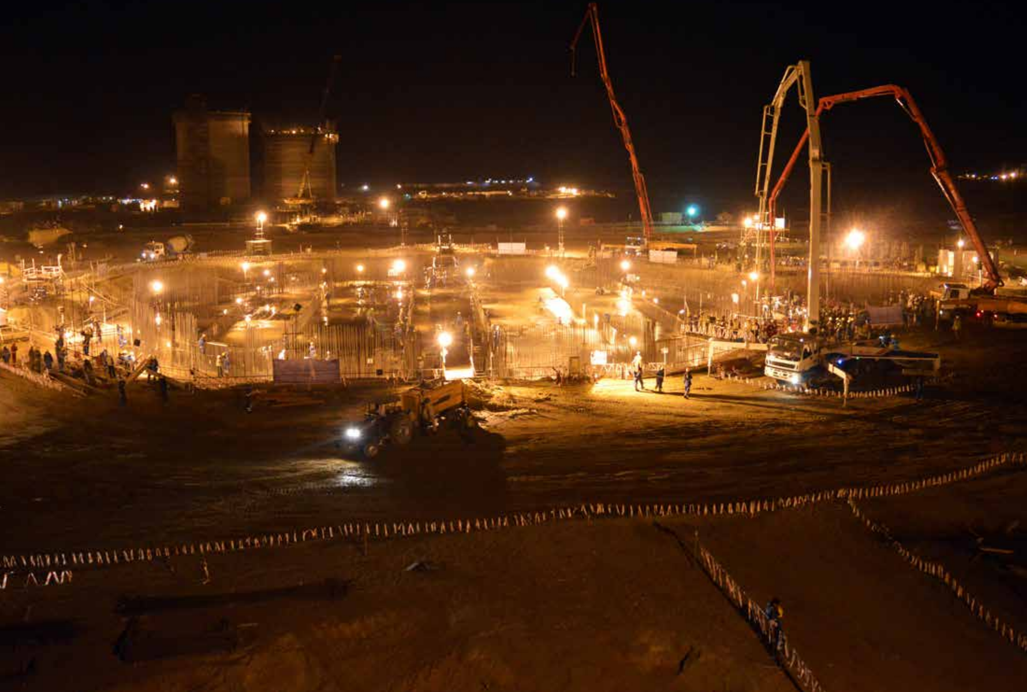
Largest Single Concrete Pour of 8000 M 3 in 48 Hrs at DG Cement, Hub, Balochistan.
